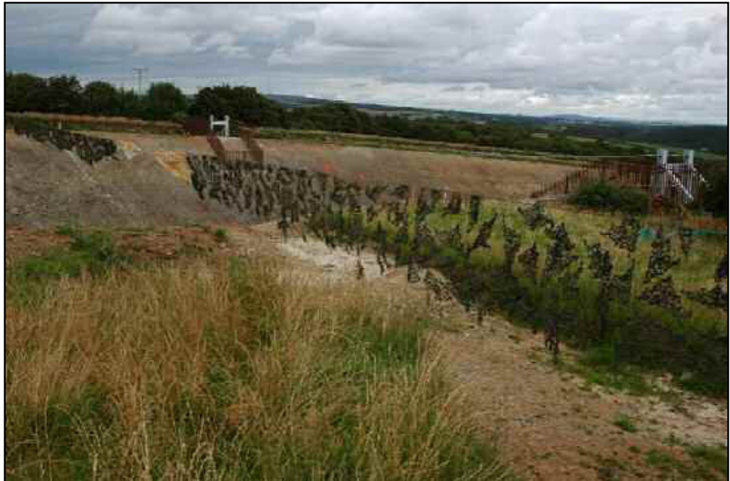
Image 1: Temporary replacement for flightline (Highways Agency, 2008)
