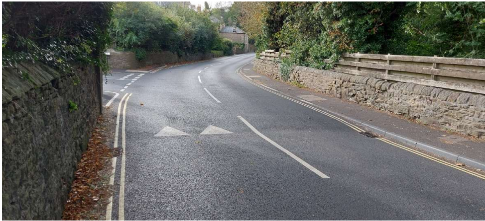
Fig. 1: New raised table layout on Allendale Road and its junction with Hextol Terrace in Hexham
