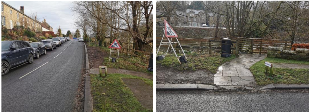
Photographs 1 & 2: Damage to grass verge at Riverside, Felton
