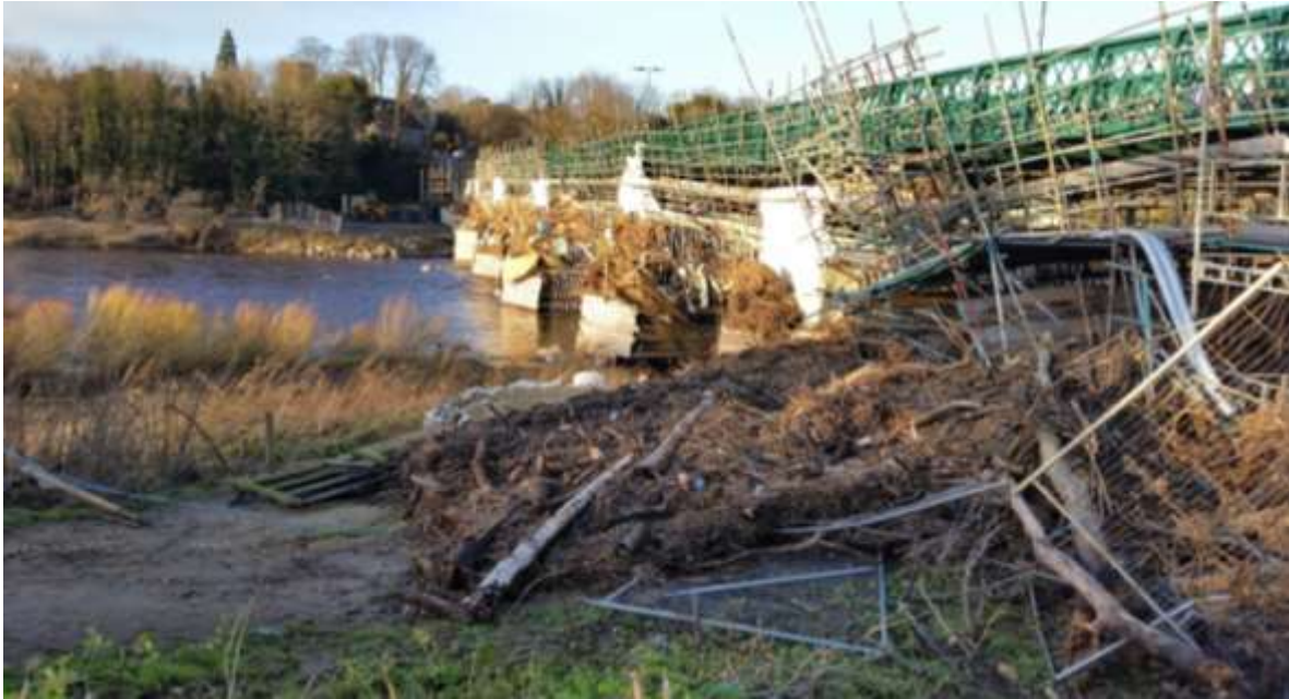
Image 1- Image of the damage dealt to the Ovingham bridge
