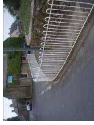
Inappropriately designed highway fencing
