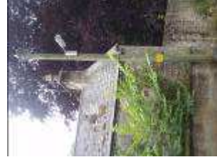
Lighting units on cable columns
