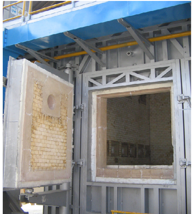
Horizontal furnace – external view
