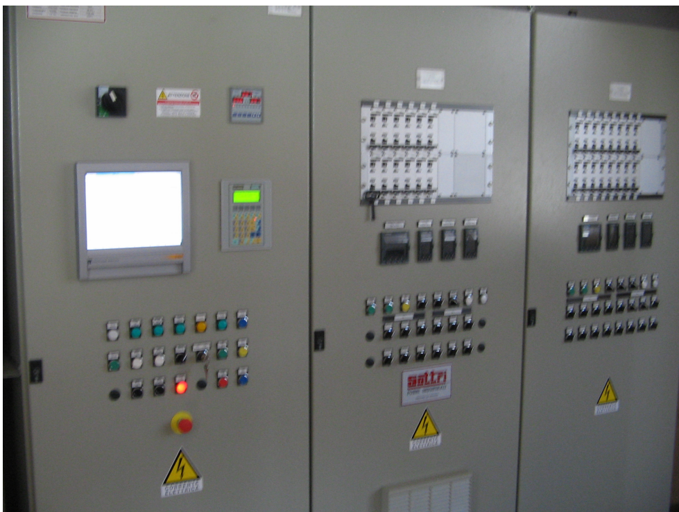
Figure 5.24 – The System Command/Control Panel for the Furnace
