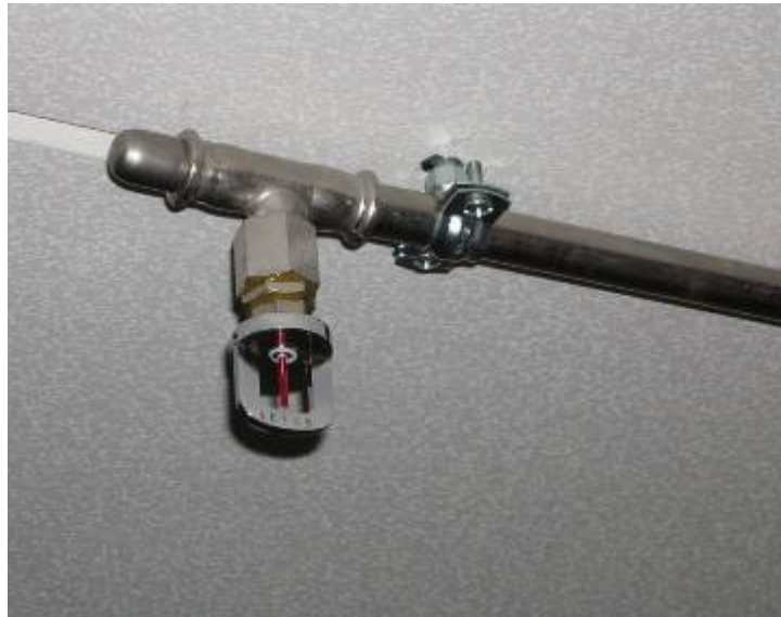
Figure 4.30 – A Sprinkler Head of a Sprinkler System Installed in a Care System in Finland
