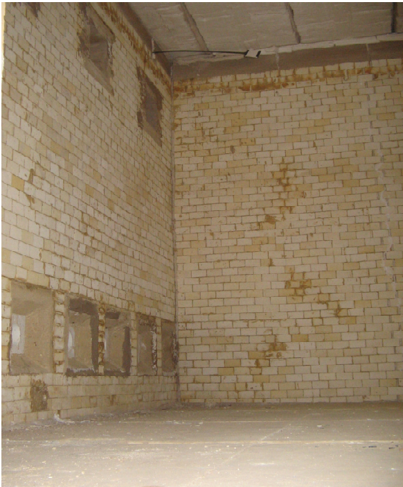
Horizontal furnace – internal view
