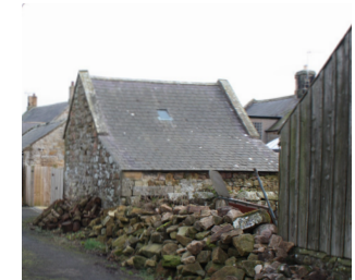
Water tabling on outbuilding
